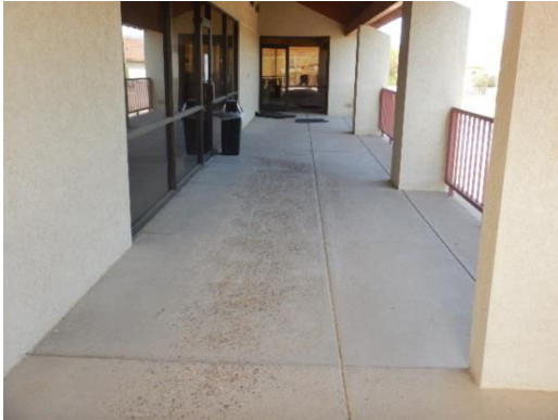
Picture of degraded concrete walk at balcony.
